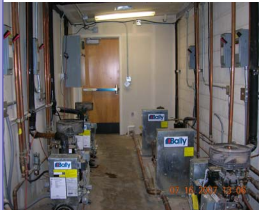
COOLER CONTROL ROOM
